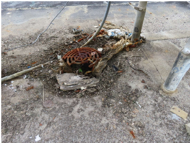
Damaged drainage grate
