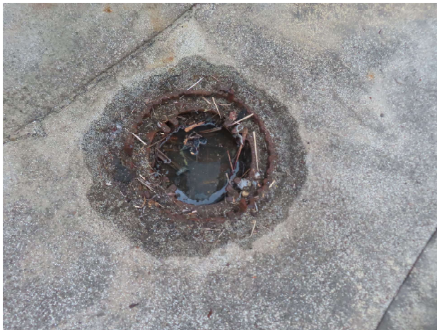
Missing grate - Plugged drainage pipe
